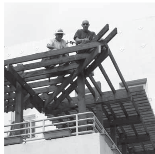
Construction workers install the trellis of the Serenity Roof Garden generously donated by the Solid Rock Foundation.
